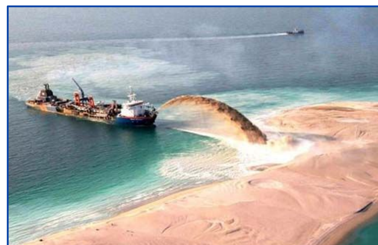
Figure 2: Redeposition of sediment and sand in progress to construct Palm Jumeirah artificial islands. The project, completed in 2006, totalled $12 billion USD in costs.
